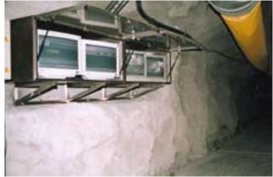
The control center with its monitors.
