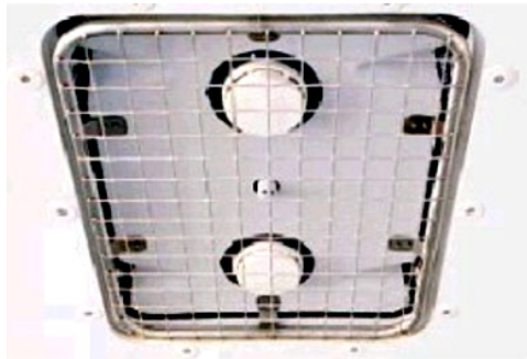
Figure 1: Two smoke detectors in a cavity for installation in the ceiling of a cargo compartment
